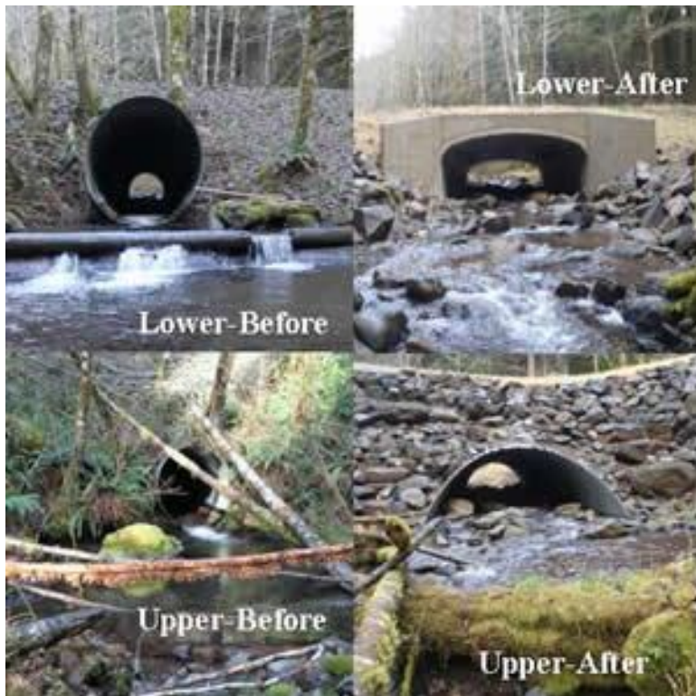
Figure 4. Fan Creek Culvert Replacement: This project, funded by the BLM and OWEB, replaced two passage barrier culverts on Fan Creek, a tributary in the upper Nestucca River watershed.
